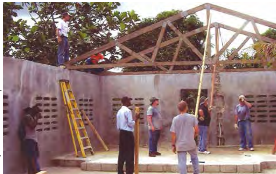
The Illinois church team at Plain de Nord church site, hoisting roof trusses into place.
